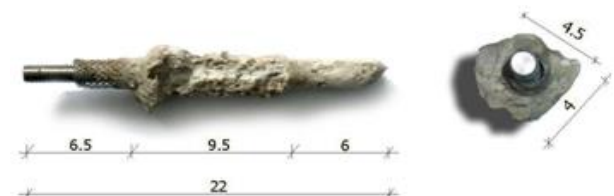
Fig. 7. A view of destruction fixing anchor with concrete substrate.
